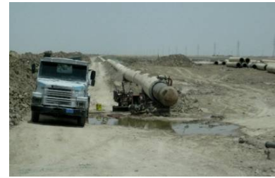
Oil piping networking
